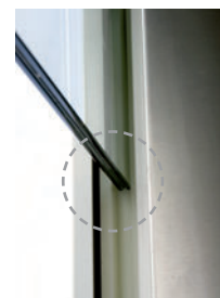
Window not sealed
